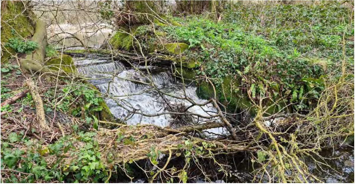
The cascade to Island Pond is functional but leaking.
