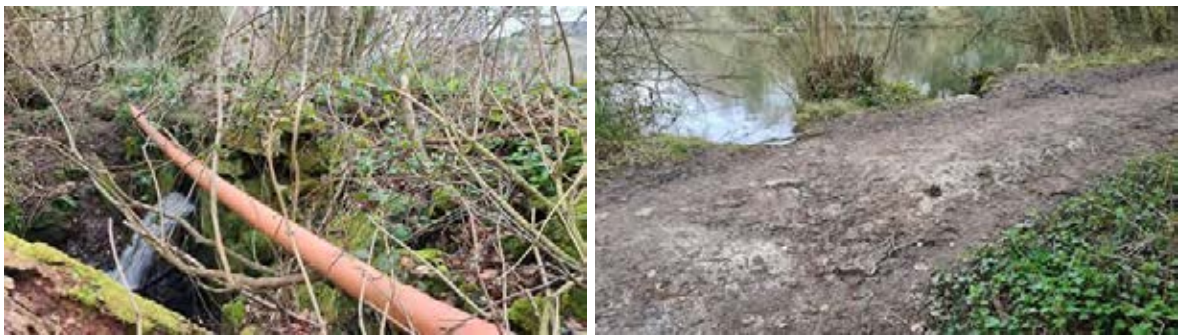
Left: the outfall (the flowing water) of Pale Park Pond is too high and/or too small. Right: evidence of overtopping on Pale Park Pond Dam.
