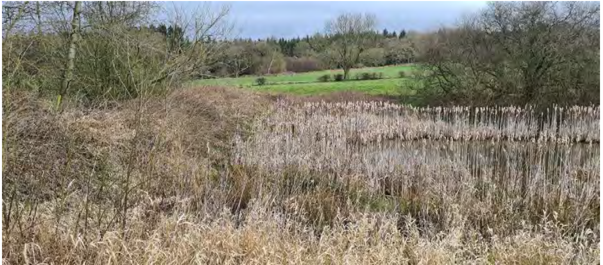
Creswell's Pond embankment. Low water level and extensive vegetation both reedbeds and woody scrub/trees
