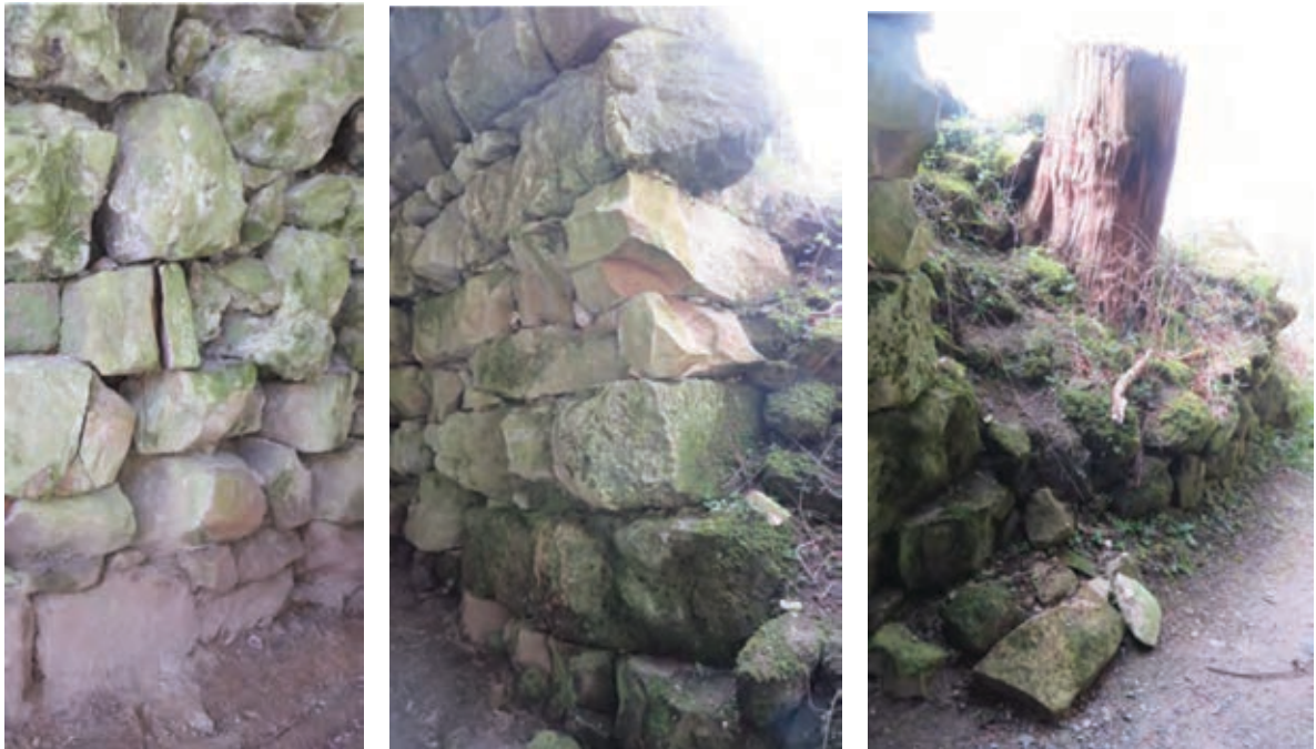
Left: a section of the support wall on the south side of the barrel vault – note the series of vertical fractures and some adjacent voids. Centre: the west end of the support wall at the point where it should extend as a wall is now much lower – note the fractures and losses of stonework. Right: a section of the adjoining wall is considerably lower than it must have been originally and is now pushed out by a tree which had been felled by 2011.
