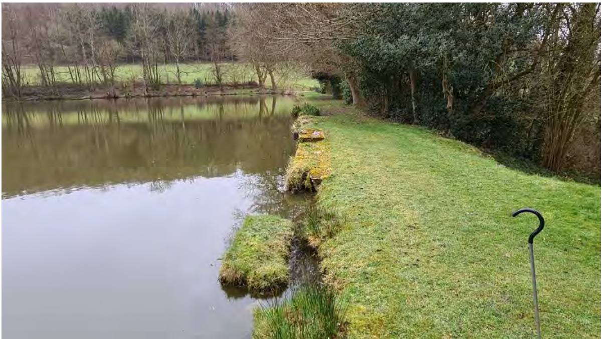
The collapsed and slipping dam wall stonework viewed from the north.
