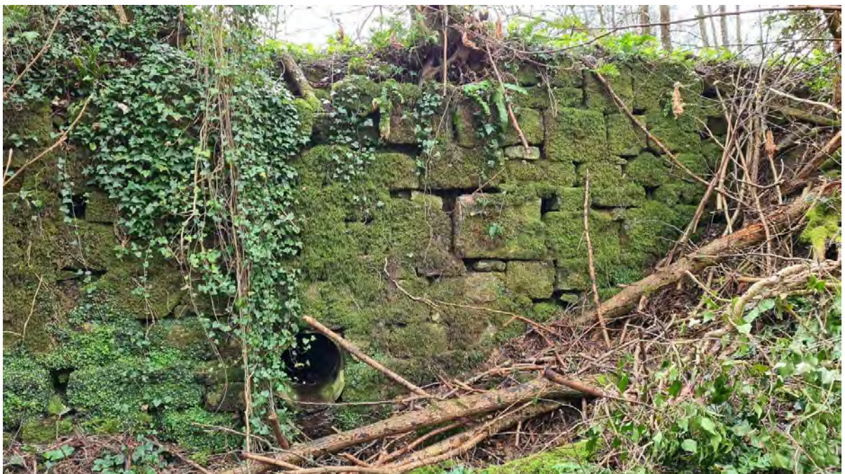
Scour outlet headwall at Pale Park Pond has moved, most likely due to root heave.
