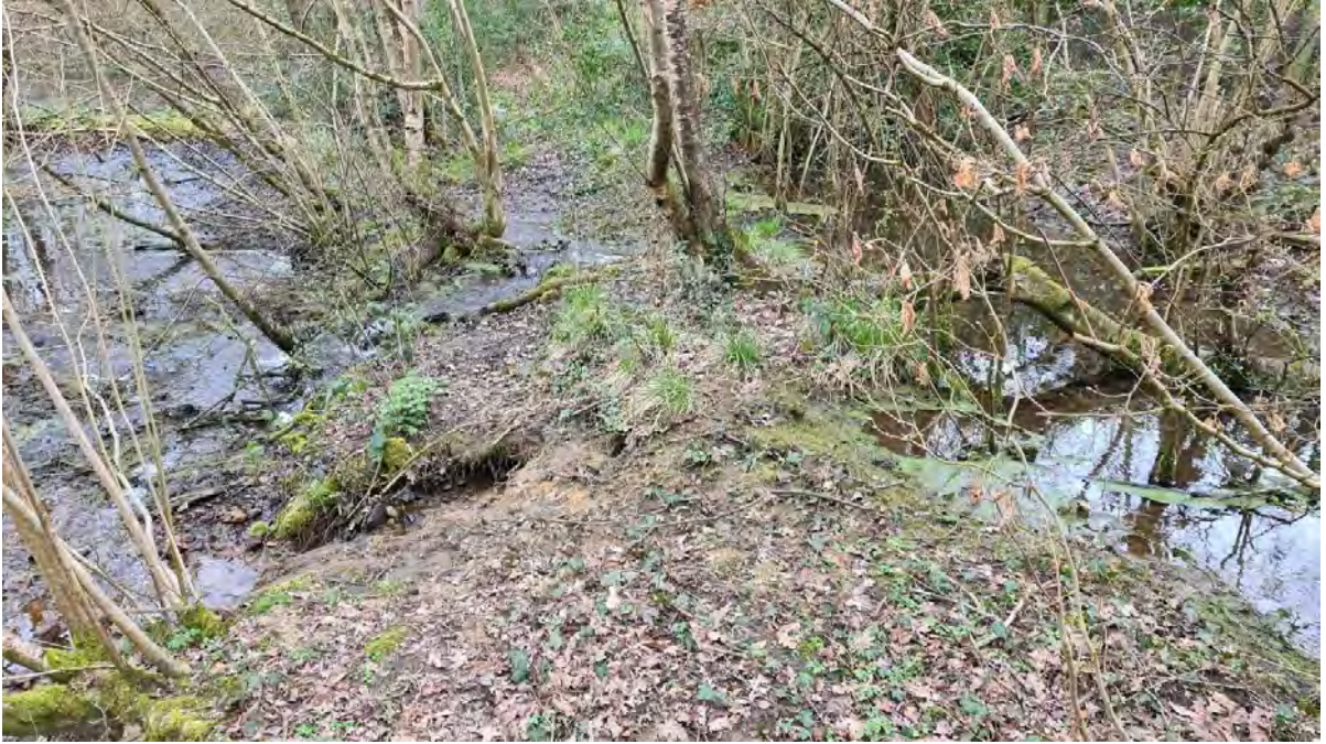
The impounding structure of Close Pond with the immediate upstream part of the Pale Park Pond to the left. Multiple leaks and evidence of regular over-topping.
