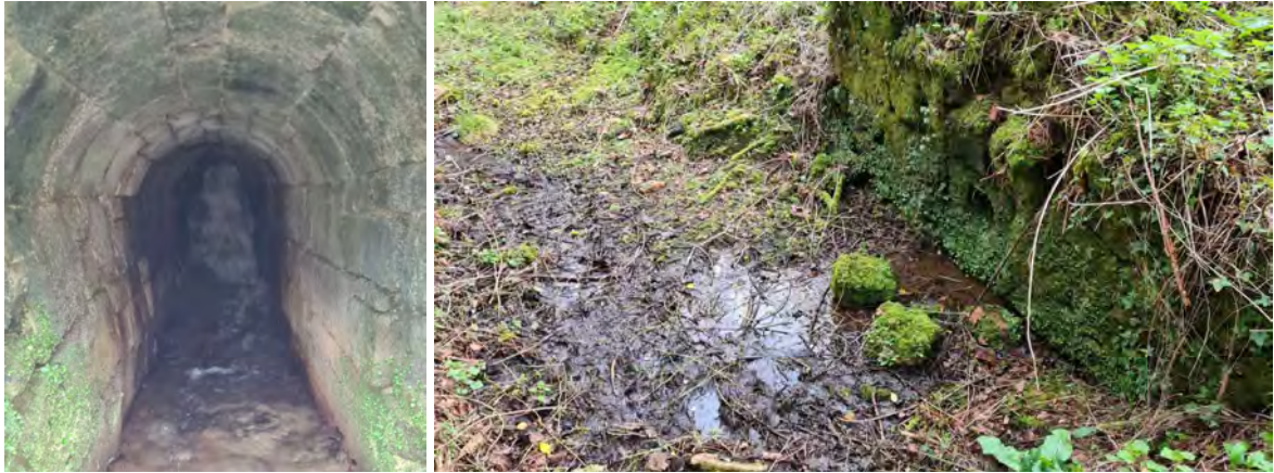
Left: the culvert in the dam is in reasonable condition, but traffic over the dam should be restricted and the bulging wall monitored or repaired. Right: Lake seepage through the dam in and around the scour outlet head wall.
